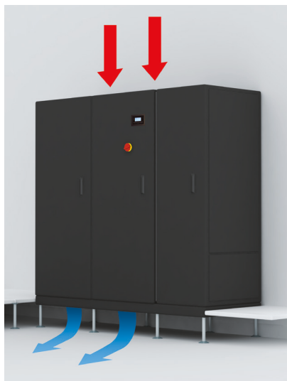
Standard version with top air intake and downflow air supply, with stand for raised floors.
