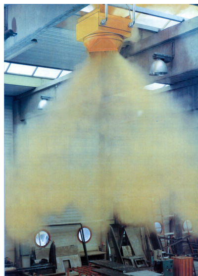
Air distribution with RotaVent
